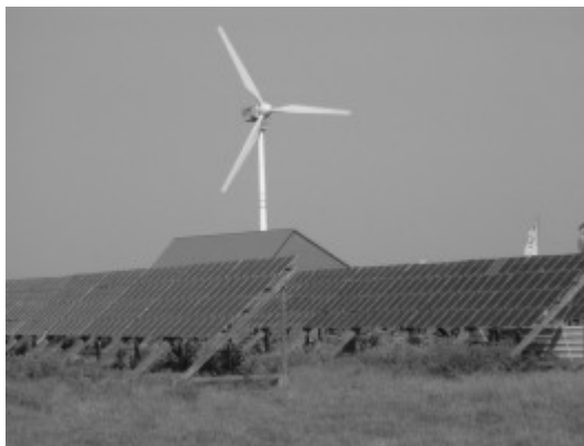
Figure 1: PV generator on the German island Pellworm
